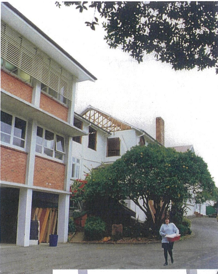
Left: The Demolition of "Old" Convent in 1998. A new convent had been built on Kitenui Ave as Integration would have put the sisters in the middle of the school and unable to have their property delineated. The "old Convent" no longer met building code requirements.
