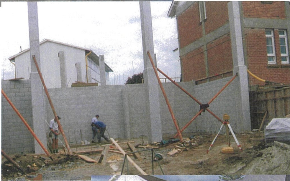
Below: The view from Alberton Ave during construction. Note the original high school building still stands and was used as an art room until the Juliana Library and Information Centre and art room were built in 1999.
