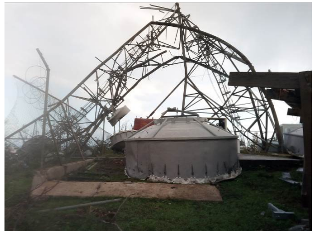
Digicel tower at Lalwori
