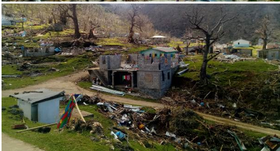
Views around the mission showing damage to houses
