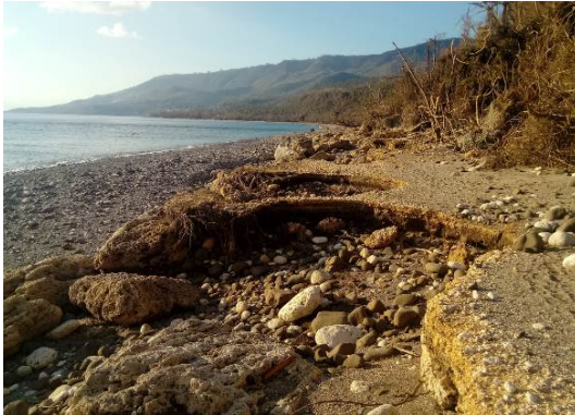
Parts of the road between Melsisi and Lonorore Airport that were damaged by the sea
